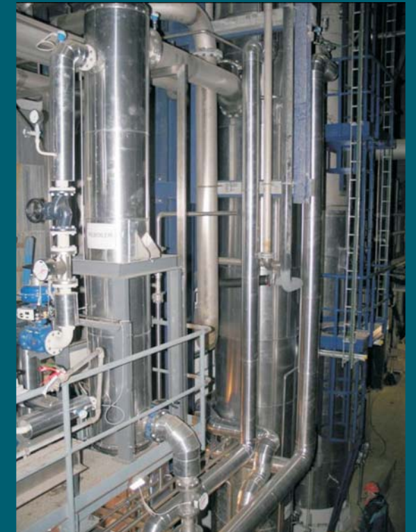
The 1 t/hour CO 2 capture pilot plant using an amine wash process that is installed at the Elsam Esbjerg power plant in the framework of the EC CASTOR project (courtesy of IFP)
