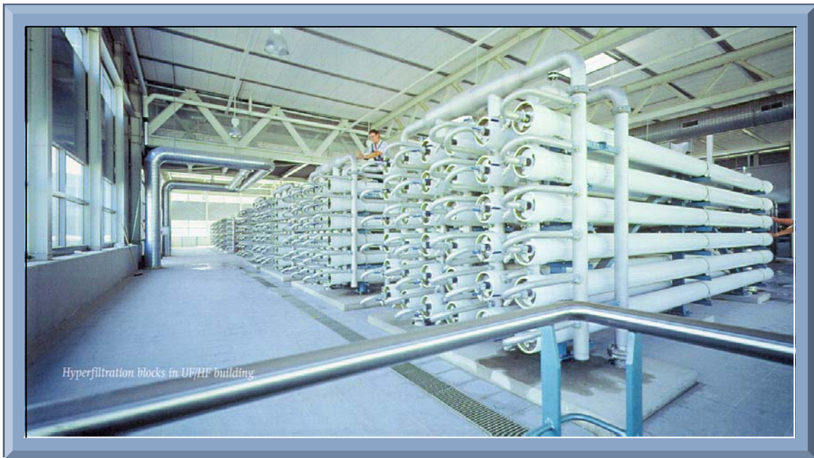
Membrane filtration installation in drinking water production. PWN the Netherlands
