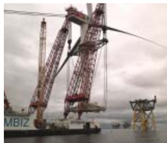
The Beatrice WTG A (Wind Turbine Generator Alpha) being lifted onto its jacket substructure, with Beatrice A oil production platform in the background.
