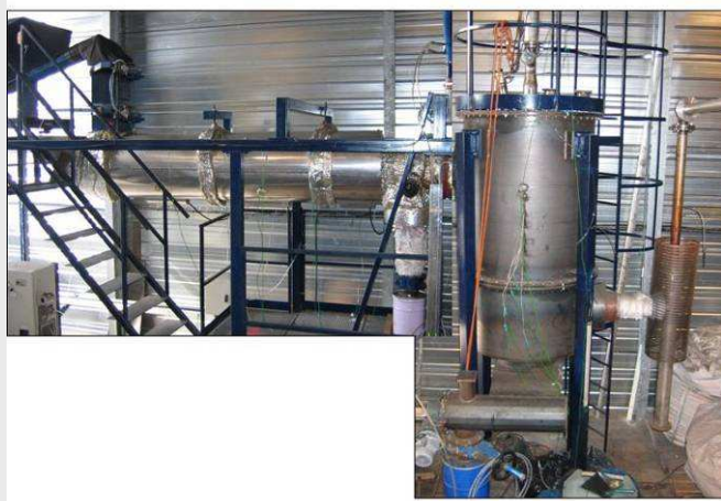
75 kWth (20 kg/h) stage gasifier
