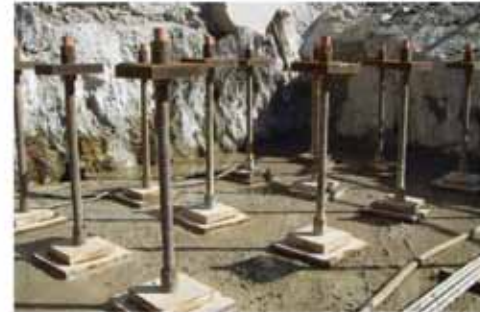
SAS Micro piles for the Foundation of new World Trade Center in New York
